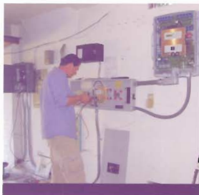
The backup system involves much more complex wiring than standard solar systems.
