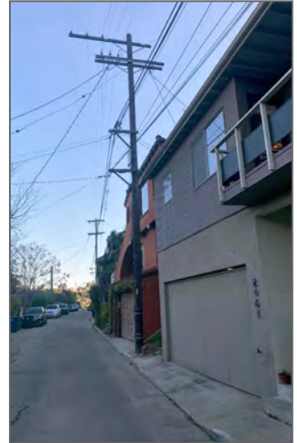
POWER POLES WITH DW&P HIGH VOLTAGE LINES ON THE TOP TWO CROSS ARMS AND TELEPHONE AND CABLE LINES ON THE BOTTOM TWO CROSS ARMS
