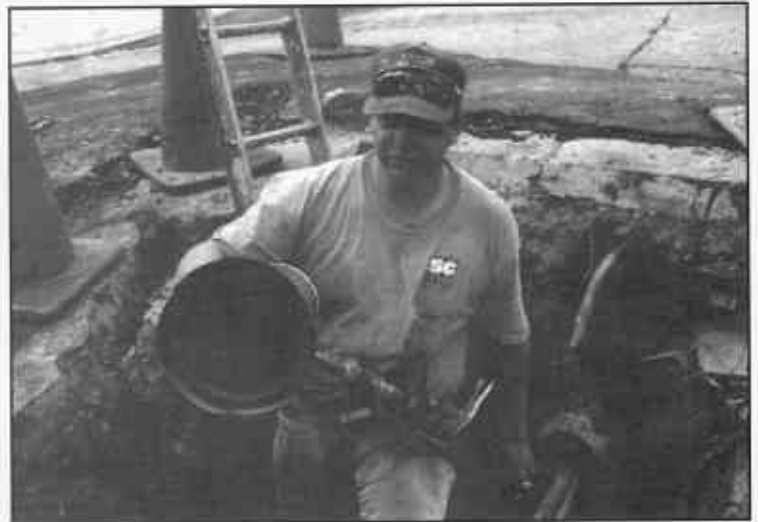
It's a messy job but . . . David Trujillo prepares the cement spraying nozzle and spring loaded trowel to be pulled through the 8" water main under Mayview Drive
