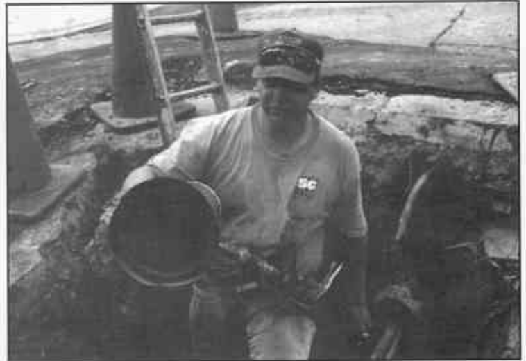
It's a messy job but . . . David Trujillo prepares the cement spraying nozzle and spring loaded trowel to be pulled through the 8" water main under Mayview Drive
