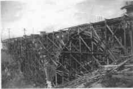
Shakespeare Bridge construction lasted from 1924 to 1926. This view is from the north side. The original construction cost just $59,960. The 1997-8 seismic strengthening cost over 2500% more—about $1.5million.
