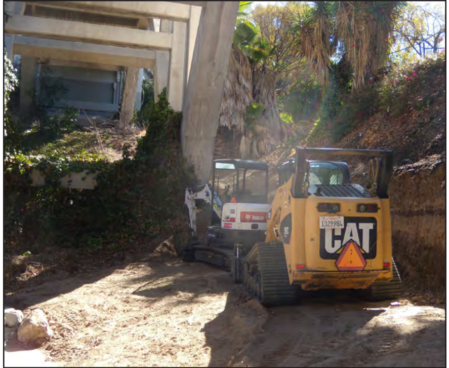
Construction work began in September. The slope has been cut back where a retaining wall will be installed.
