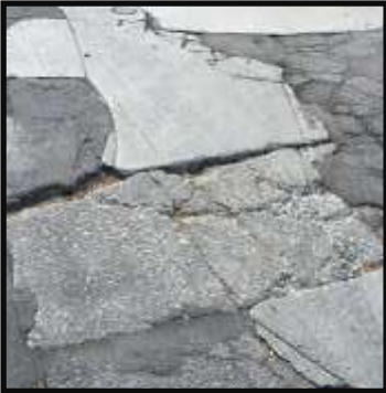
Broken concrete and asphalt repairs plague our streets (photo by Chris Boutelle).
