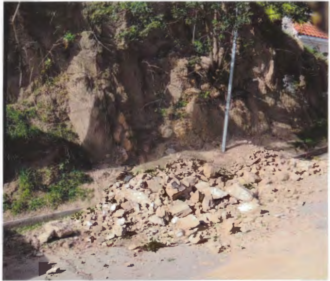
ABOVE A strong wind storm in 2012 loosened tree roots and caused this part of the hillside on Lyric Ave. to fall into the street.
