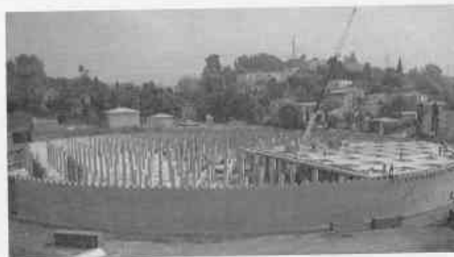
DURING: 10 million gallon concrete tank under construction. Inside, before it was filled with water, it looked like a very high ceiling parking garage.
