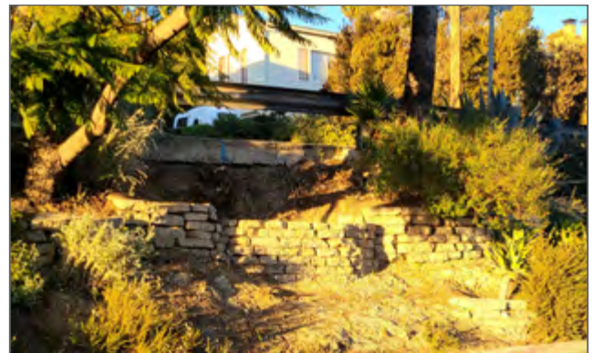
SECTION OF THE SHAKESPEARE BRIDGE MEDIAN GARDEN IN NEED OF REPAIR.
