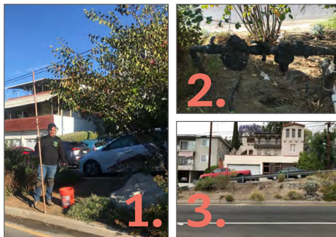
1) REPLACING THE GATE VALVE 2) THE BACKFLOW PREVENTER AND PRESSURE REGULATOR 3) BARE SPOTS BEFORE INFILL BEGAN
