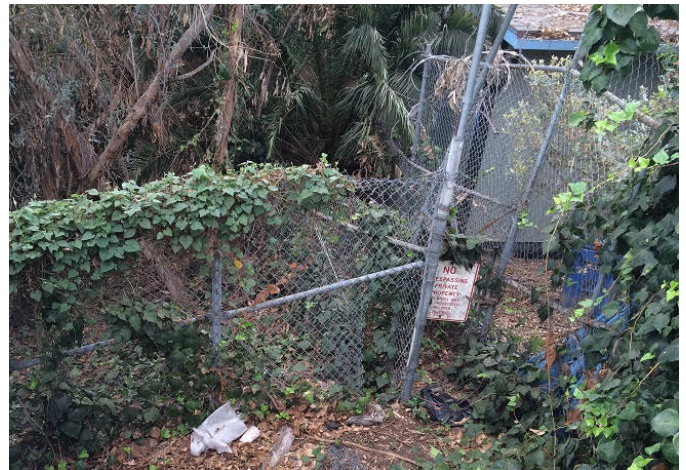
Fencing that was cut where people were dragging down trash and furniture under the west side of the Shakespeare Bridge. Photo by Rachel Fox.
